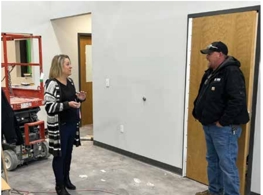
Chrissy Simmons, executive director for Bright Beginnings and Maslow Academy, discussed completion plans with Tony Vroman, field superintendent for Shaw Construction, the general contractor who worked on the new location for the infant and toddler school at the Colorado Outdoors Campus. (Stephen Woody/Special to the MDP)
